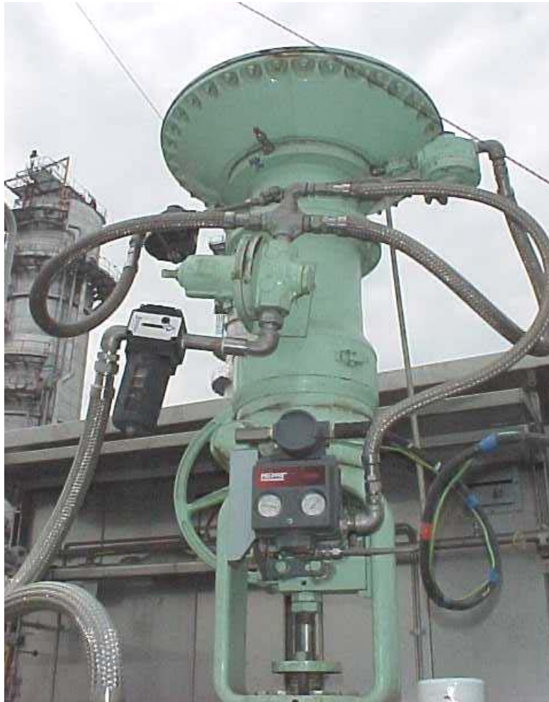
XFV-026 Pumparound Control Valve
